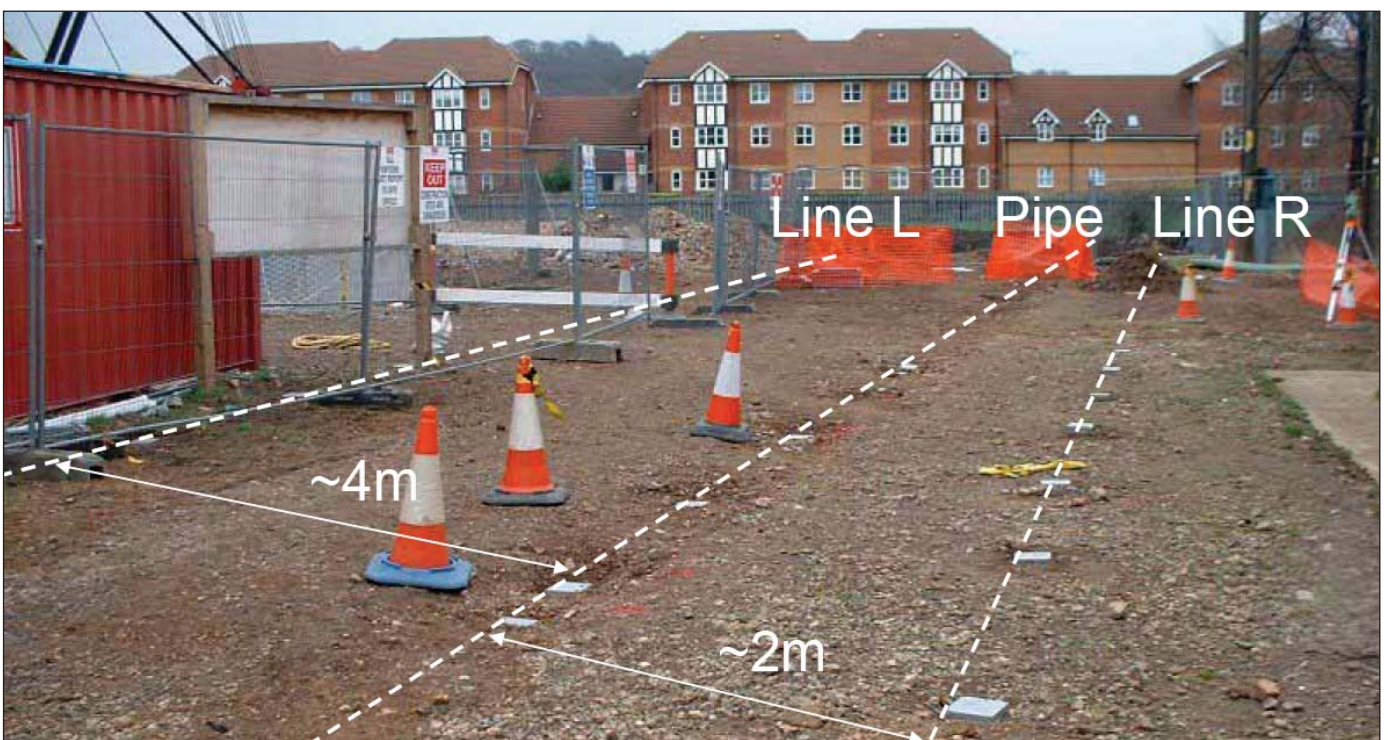
Pipeline and BOTDR positions at Chingford.
